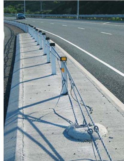
Wire-rope barriers - minimising initial cost at the expense of safety.
