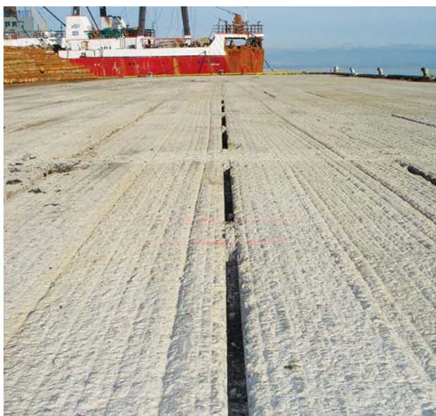
Kingsford Quay Wharf - desired surfaced texture for effective bonding.
