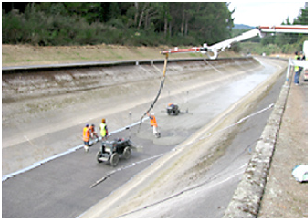
Re-lining the Poutu Canal – the driving force behind the Tokannu power scheme.
